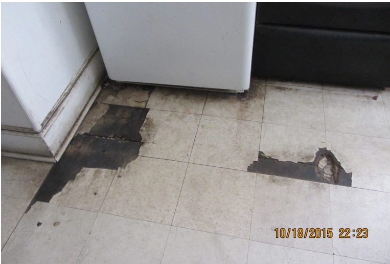
Worn kitchen floor
