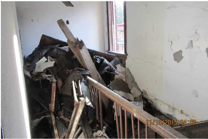
Stairway blocking entrance to the 3rd floor
