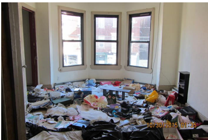
Front bedroom—typical of the debris inside the building.
