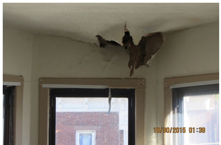
3rd Floor ceiling showing roof damage
