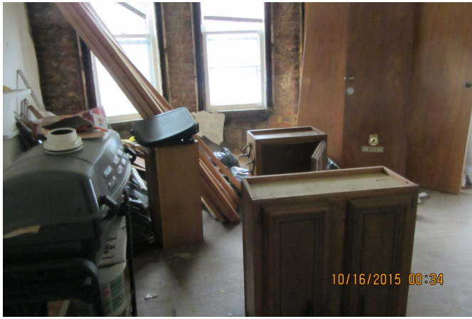
1st floor gutted room
