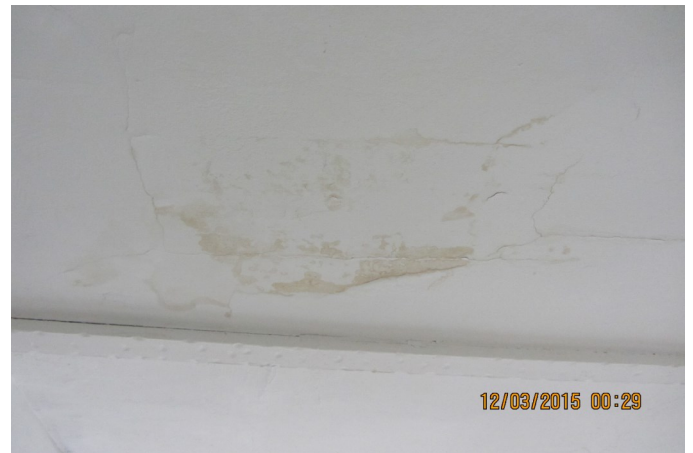
Interior leak marks
