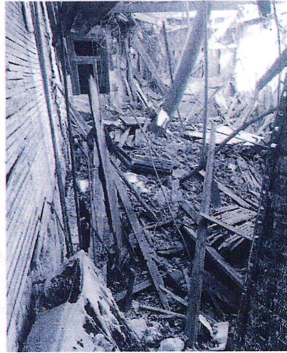
Interior Building Components/Debris (Typical)
