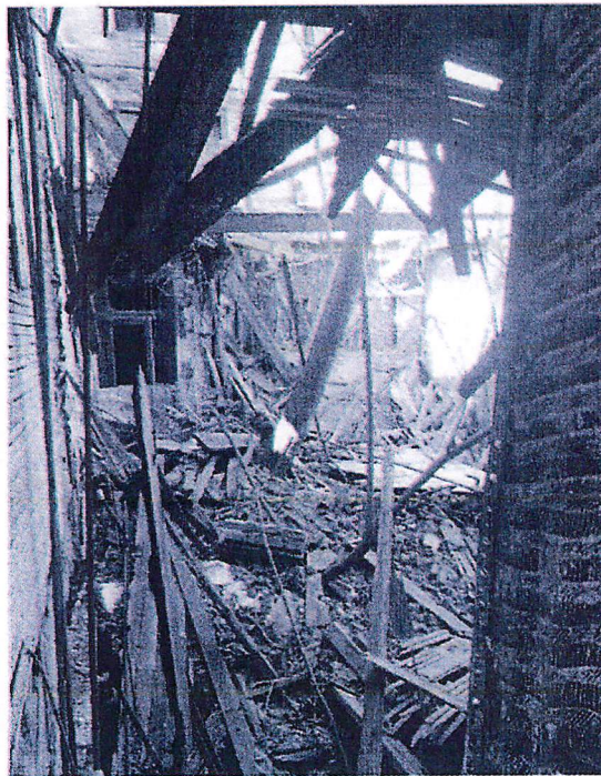
Interior Building Components/Debris (Typical)
