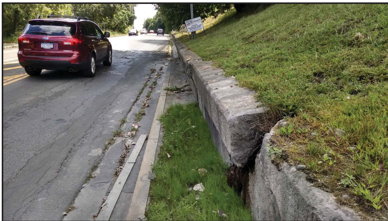
Figure No. 4: Severe rotation of retaining wall. View looking south along Marine Drive.
