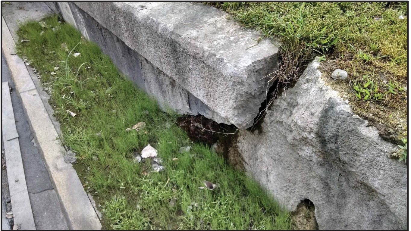
Figure No. 5: Retaining wall exhibits signs of cracking, spalling, rotation and sliding. View looking southwest along Marine Drive.
