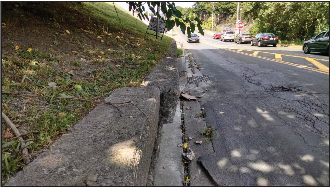
Figure No. 7: Severe rotation of retaining wall. View looking north along Marine Drive.
