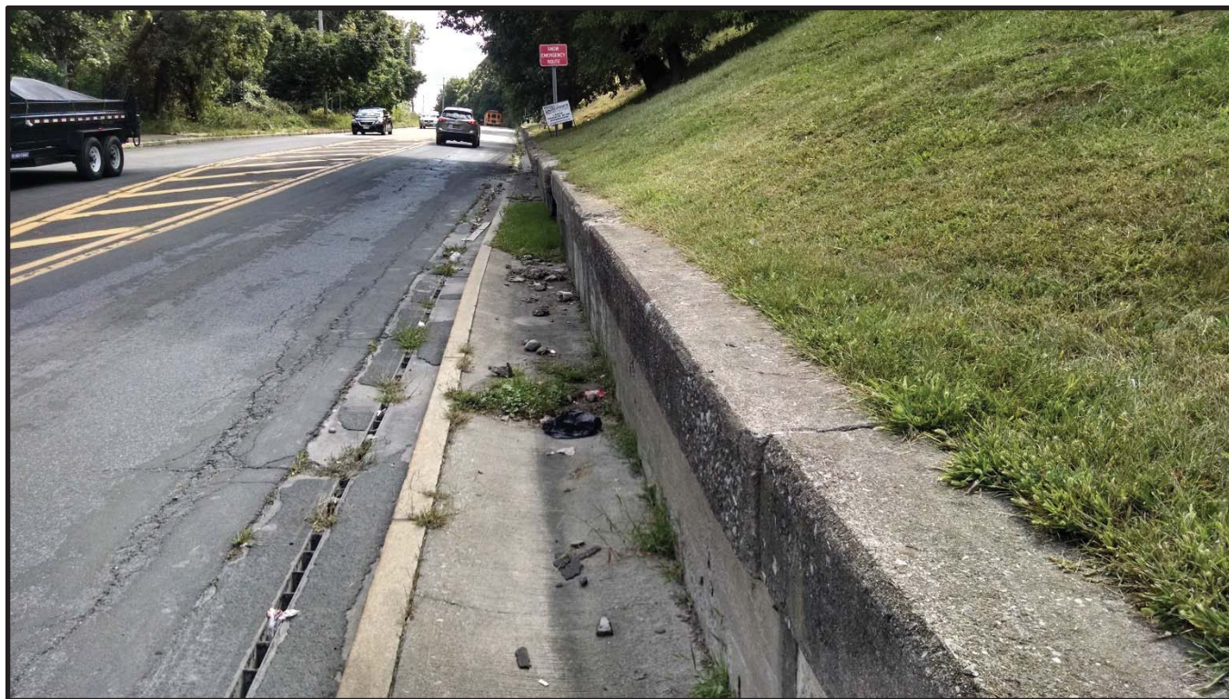
Figure No. 3: Portions of retaining wall exhibit evidence of rotation. View looking south along Marine Drive.
