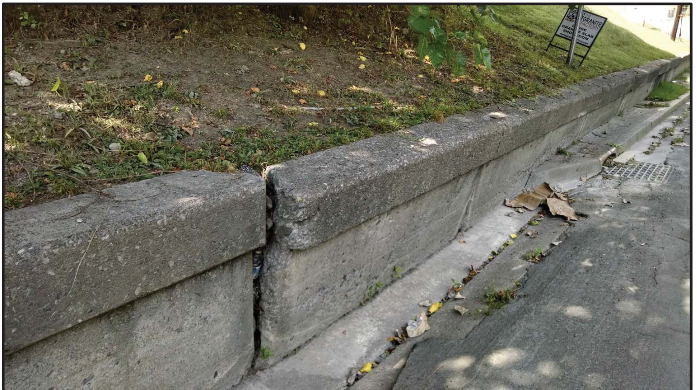
Figure No. 8: Severe rotation of retaining wall. View looking northwest along Marine Drive.
