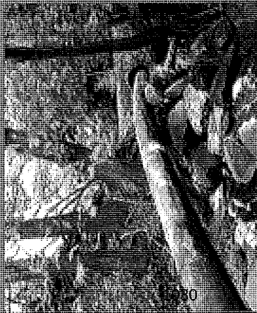
Bypass piping running down to the Quasada Creek corridor through an existing culvert to cross under railroad tracks
