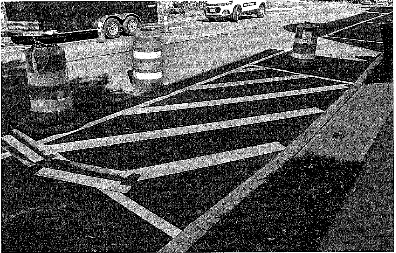
DRIVEWAY NO PARKING HATCHING EXAMPLE FROM DOWNING PARK ON THIRD STREET.
